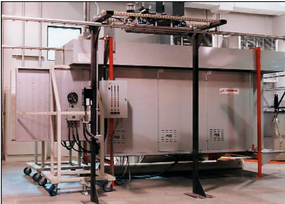
Photo 2-7: Overhead Conveyor, Infrared Oven at Advanced Energy
